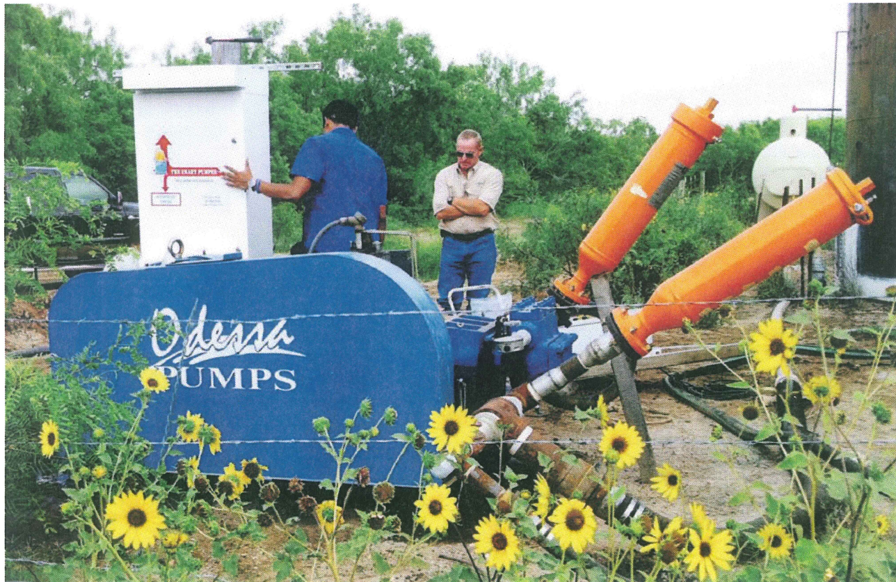
Inside the protective white box is a pump monitoring and control system called the Smart Pumper, installed in the Eagle Ford Shale. It uses fluid level data in a well to maximize production, and limit the risk of pump damage. Photo courtesy of Direct DriveHead.
